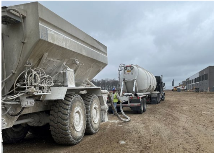
Figure 6. CQL Being Transferred from a Pneumatic Delivery Truck to a Spreader Truck.
