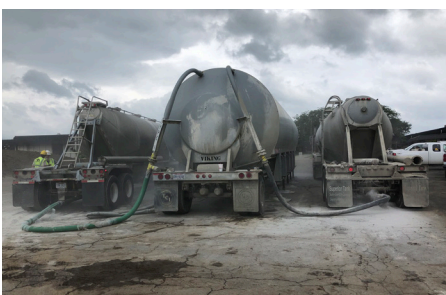
Material being transferred from two pneumatic trucks to the onsite storage PIG
